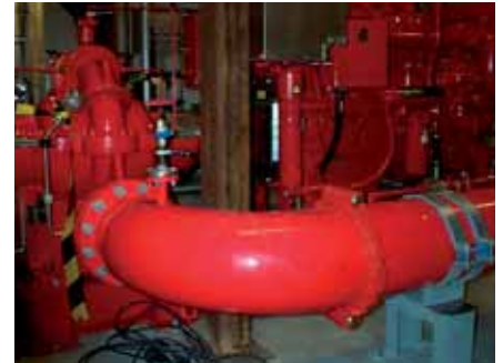
Alvenius® Thermoplastic Coated pipes are used in the fire protecting system at Ringhals nuclear power plant, Sweden.
